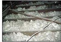
Loose fill asbestos insulation in the ceiling of a home
